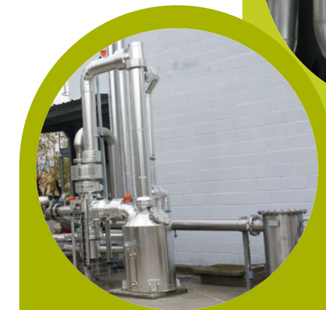
Outside water vapor removal
