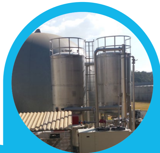
Overview of the plant
