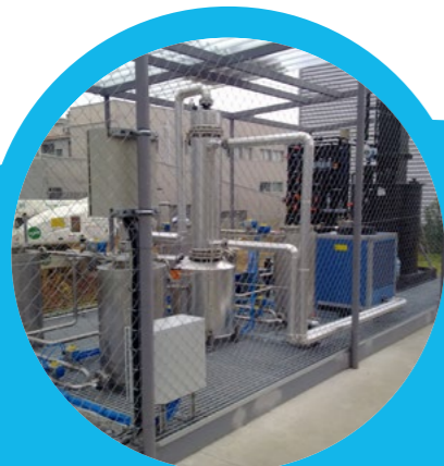
View of energy recovery.
